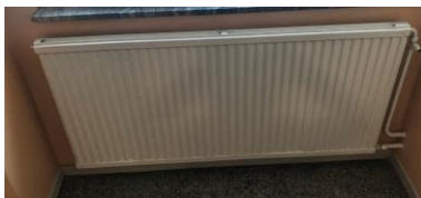
Figur 10: Trapphusradiator utan termostat
