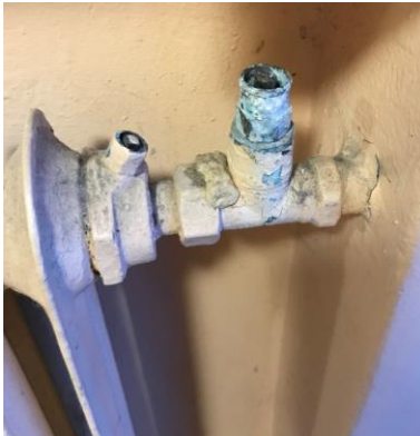
Figur 11: Trapphusradiator utan termostad
